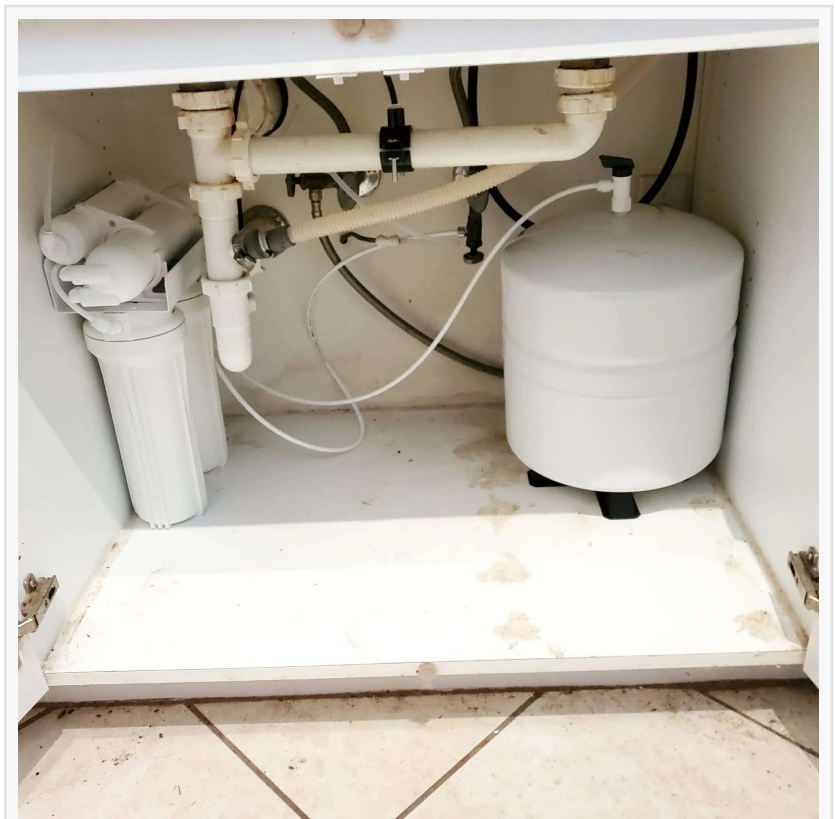
Reverse osmosis system for pure water in Port St. Lucie.
