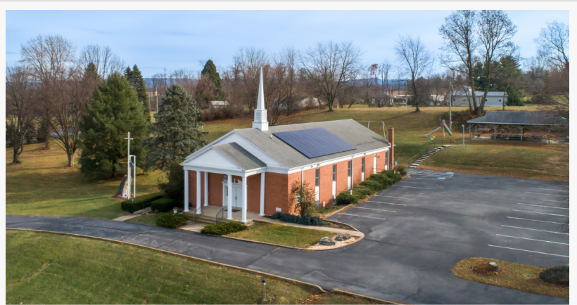
The 12 kW solar array is designed to generate 100% of the church's power needs.
