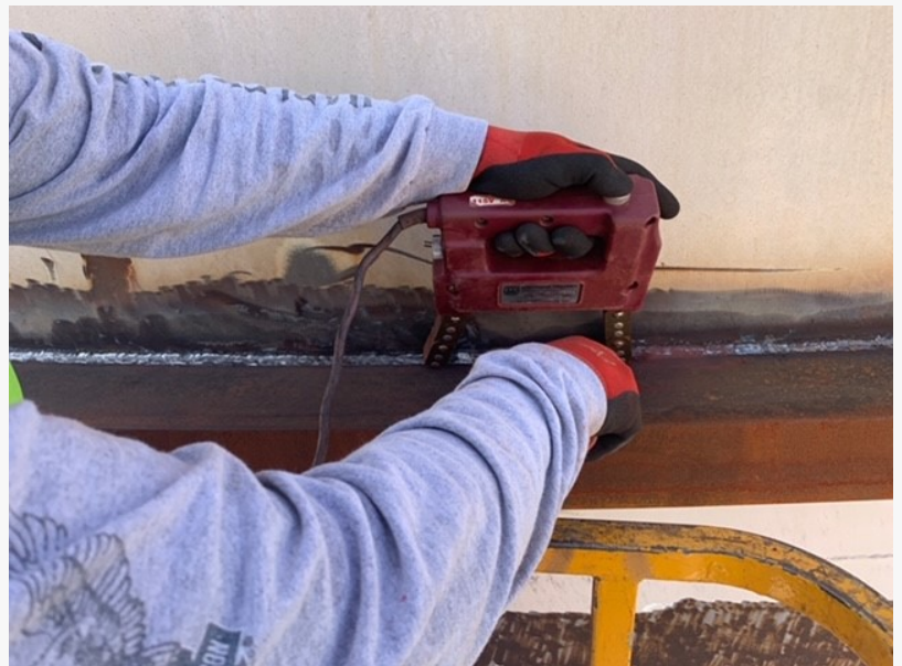
MT Non-Destructive Testing on an above ground storage tank in Long Beach, CA
