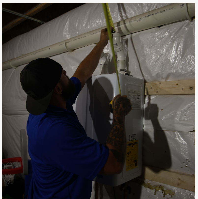
A J. Blanton Plumbing technician installs a residential water heater, helping Chicagoland homeowners prepare for winter with expert services from trusted Lincoln Park plumbing contractors and 24-hour plumbers.
