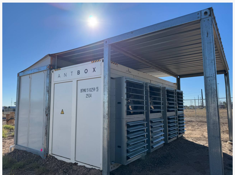
Custom Antbox Cooling System
