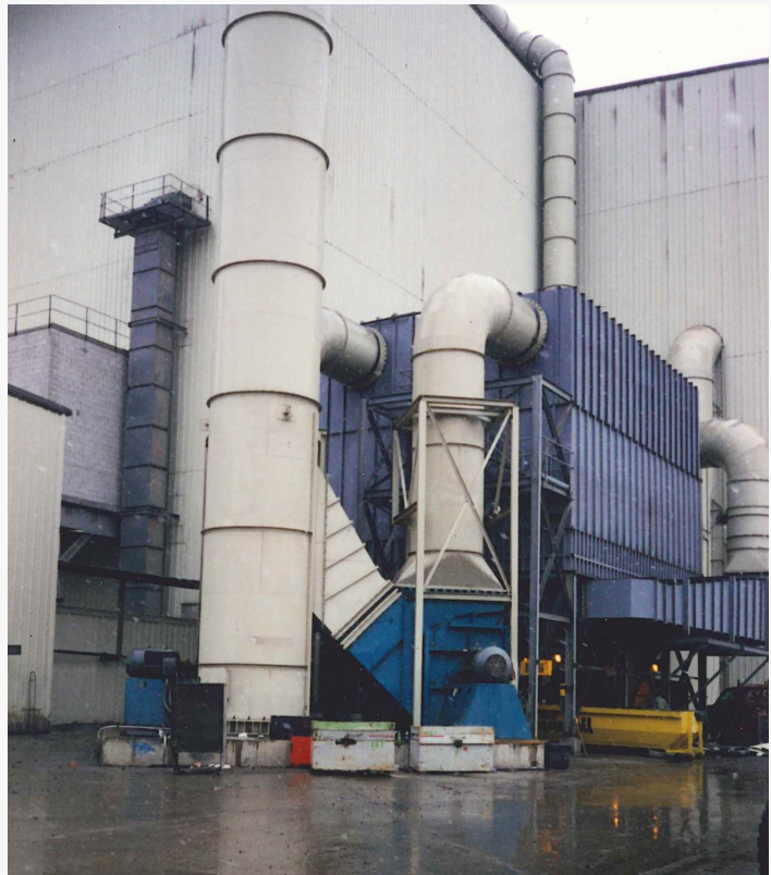
Griffin Baghouse Filter
