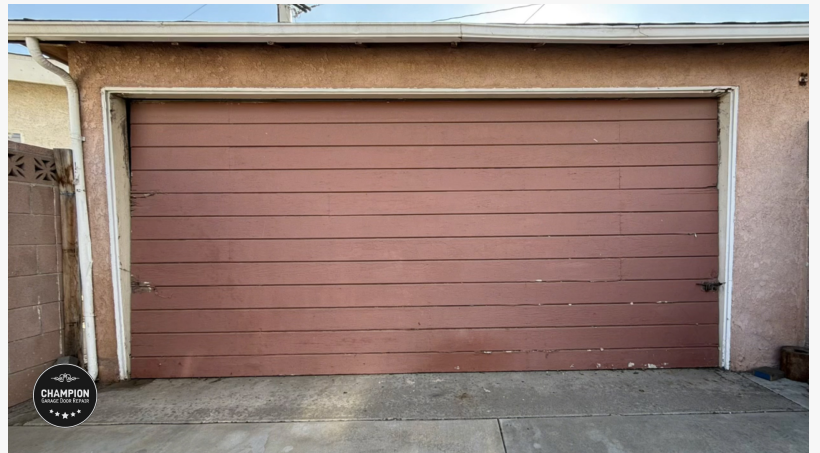
Garage Door Repair Santa Ana - Before
