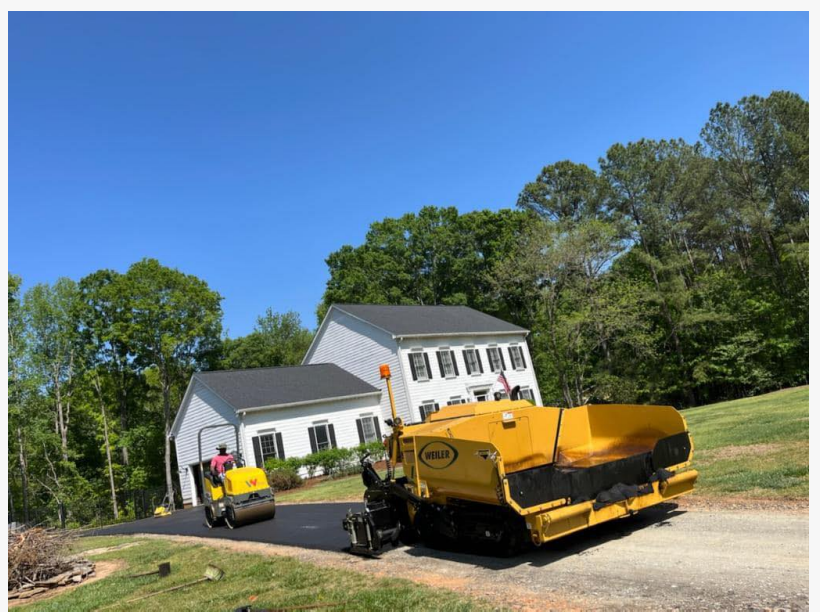
Asphalt Driveway Paving Driveway Repair in Mint Hill, NC Best Driveways Near Me
