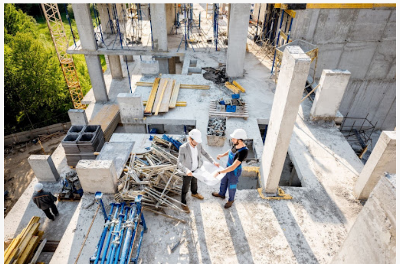
An architect reviews a blueprint while a foreman explains at a concrete construction site. In the background, partially completed structures are visible.
