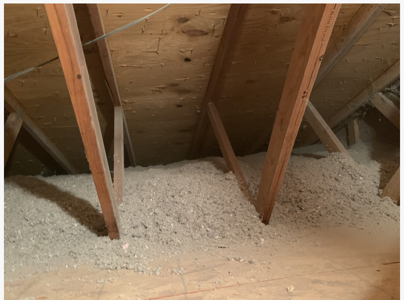
Blown Insulation in an attic
