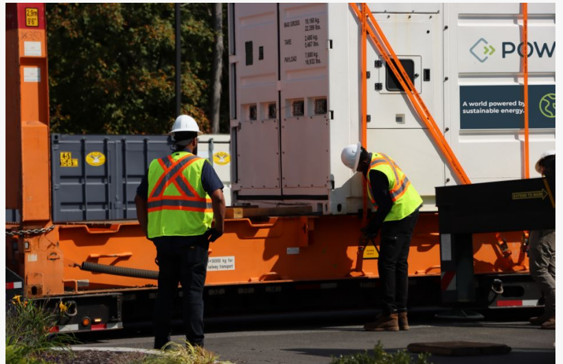
POWRBANK MAX Battery Energy Storage System
