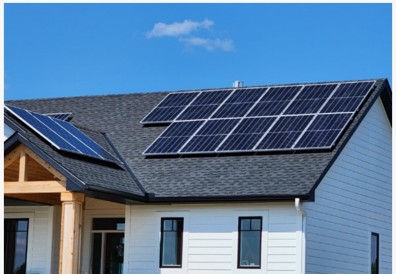
Wolf River Electric Rooftop Solar
