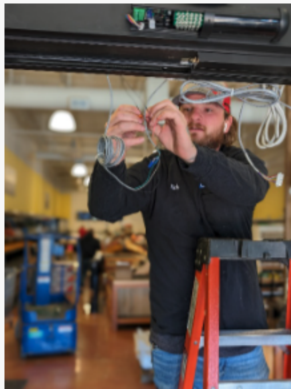
A technician expertly repairing the wiring of an automatic door to ensure reliable functionality
