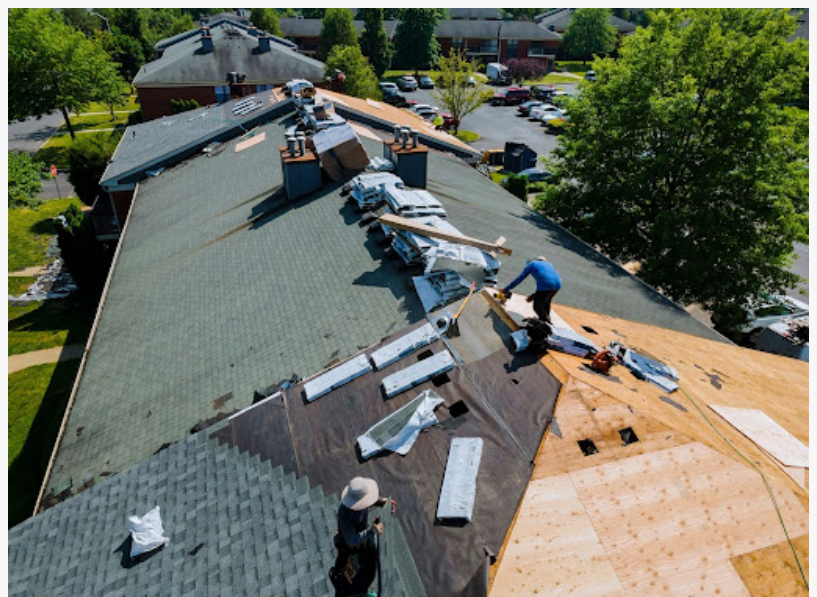
A worker providing professional roofing services while installing new shingles on a house during a renovation project.
