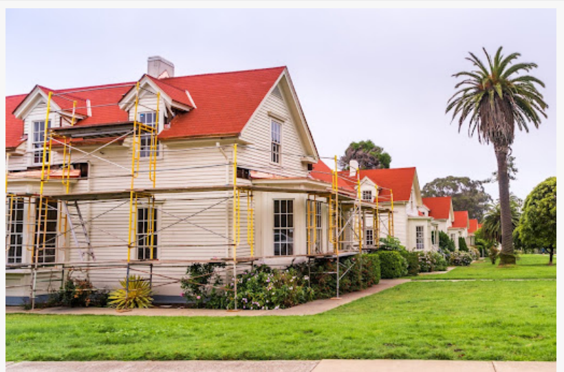
Street view of a row of identical houses, with the first house undergoing exterior renovations, including new siding and fresh paint.
