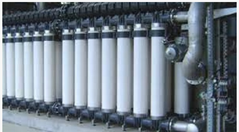
Ultrafiltration Market Overview
