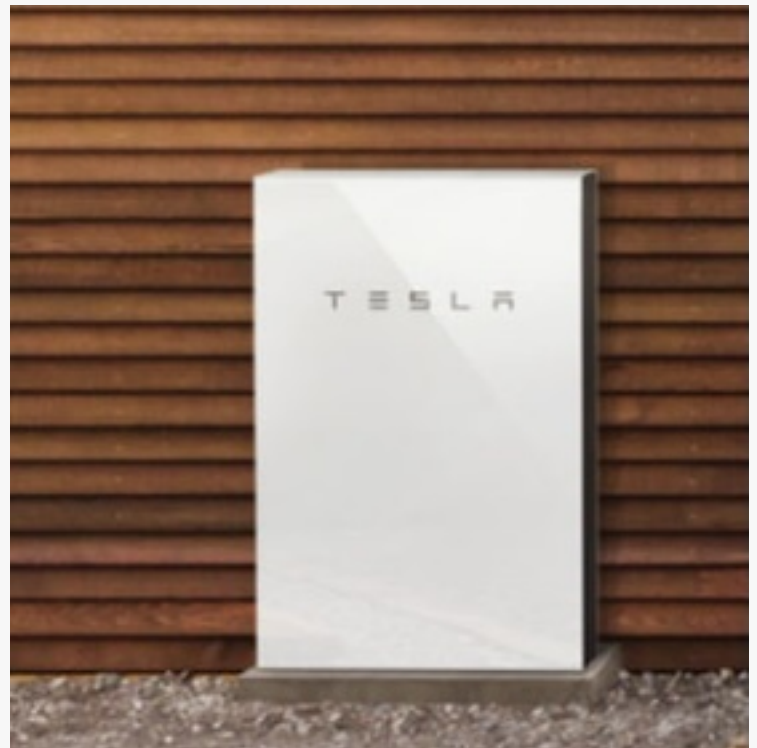
Wolf River Electric Solar Storage
