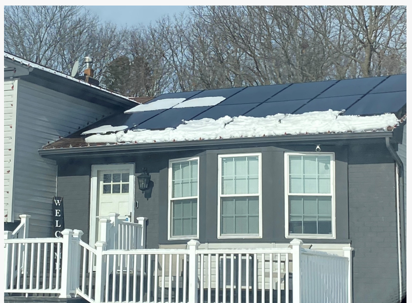
Snow on Solar Panels
