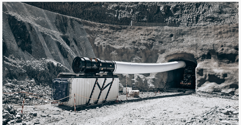
Minetek's high-performance fan at this portal provides powerful airflow, ensuring optimal ventilation and uninterrupted operations.
