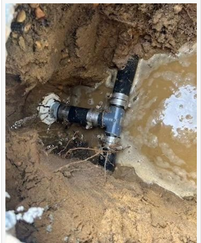
Underground pool pipe leak
