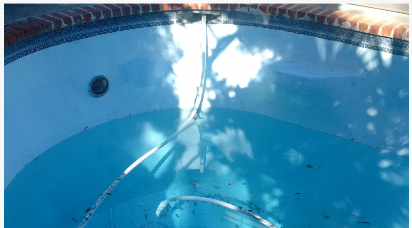
Empty Pool From A Water Leak
