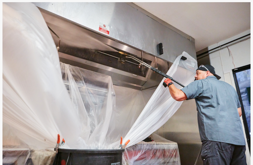
Photo courtesy of Kitchen Guard
