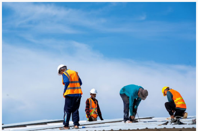
Construction workers wearing safety harnesses inspect and assemble a new roof with precision and safety.
