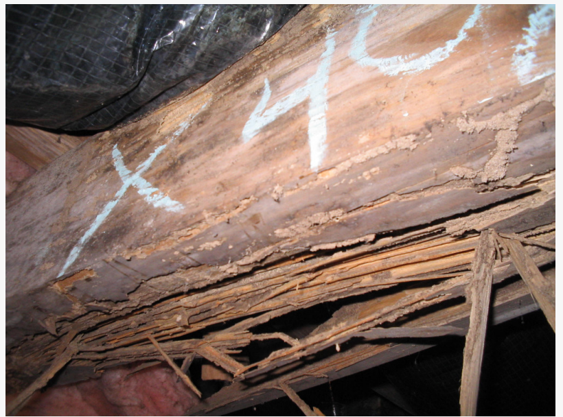
Termite Damage in Virginia Beach
