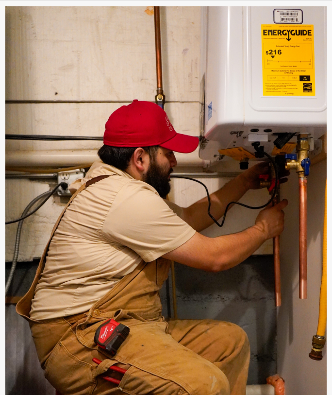
A J. Blanton Plumbing technician repairing a tankless water heater, providing expert after-hours plumbing services and gas line repair to address hidden plumbing damage caused by winter storms in Chicagoland homes.
