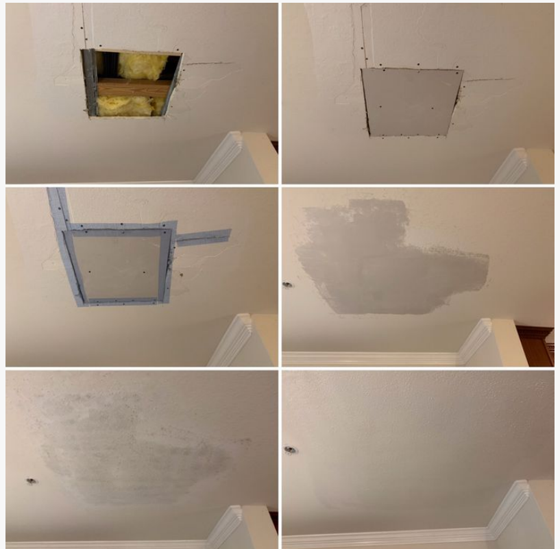
Ceiling Repair -Handyman Can Help
