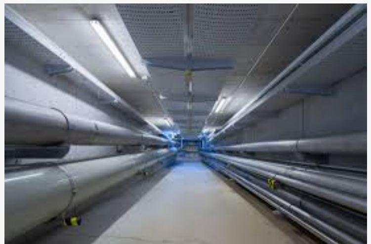
Gas Insulated Transmission Line
