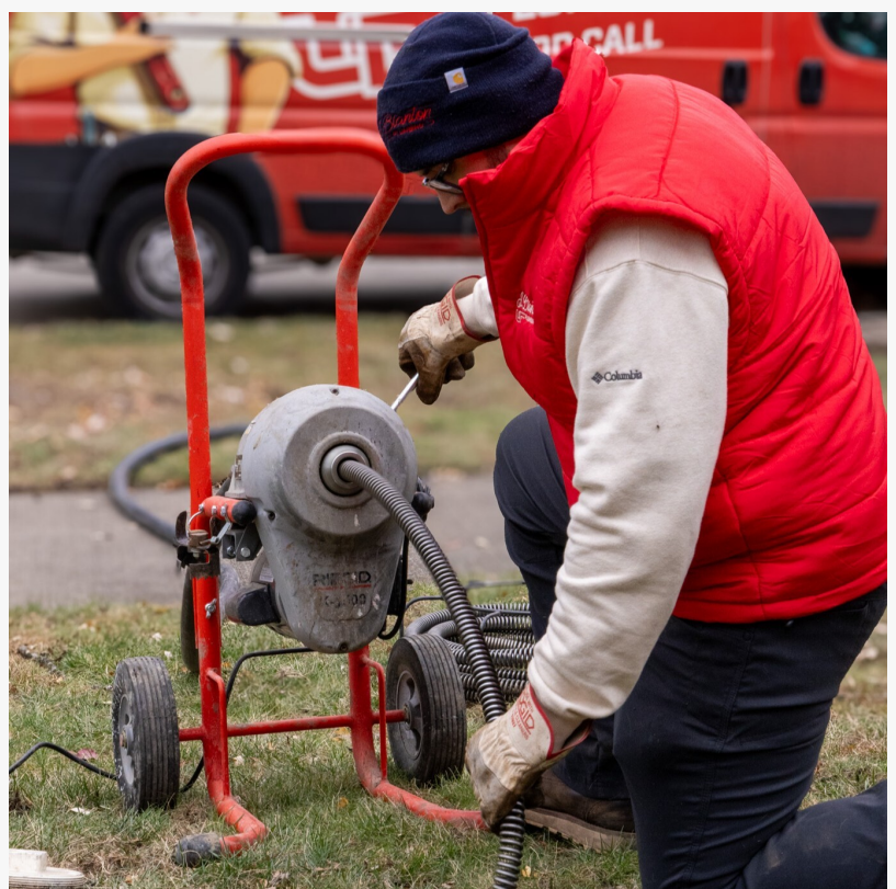
A J. Blanton Plumbing technician conducting a sewer camera inspection, helping homeowners prevent post-winter plumbing disasters with expert plumbing maintenance and emergency plumbing services.
