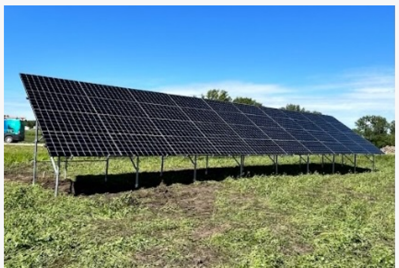
Wolf River Electric Commercial Ground Installation
