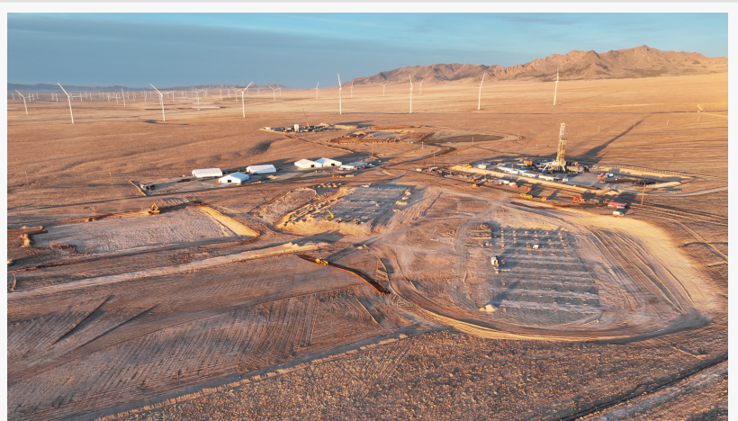
Construction site of Fervo Energy's Next-Gen Geothermal Project (Photo Credit: Fervo Energy)
