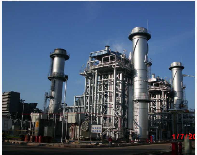
Heat Recovery Steam Generator (HRSG)
