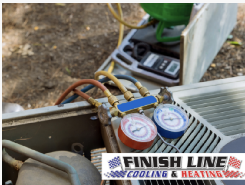
AC Maintenance - Finish Line Cooling & Heating
