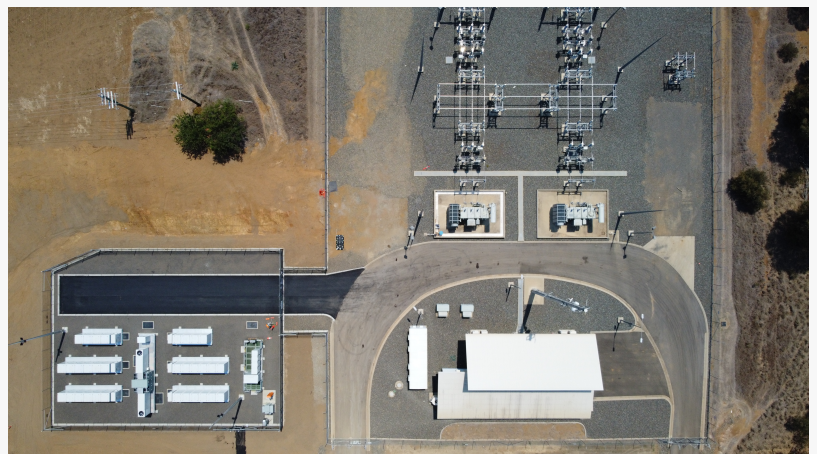
Energy Queensland Battery Energy Storage System Site
