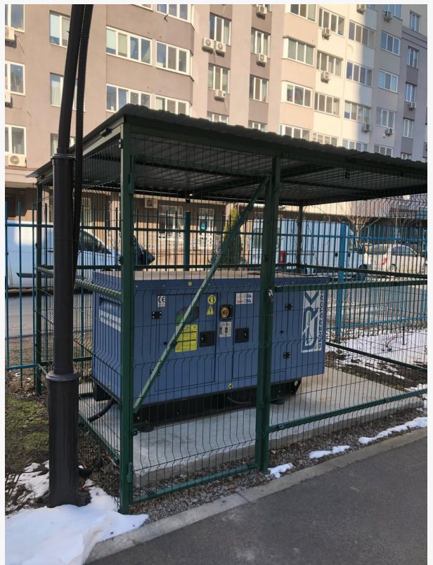
Diesel generator Vorex donated in Kyiv region
