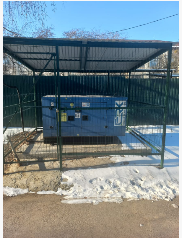
Diesel generator Vorex donated in Kyiv region
