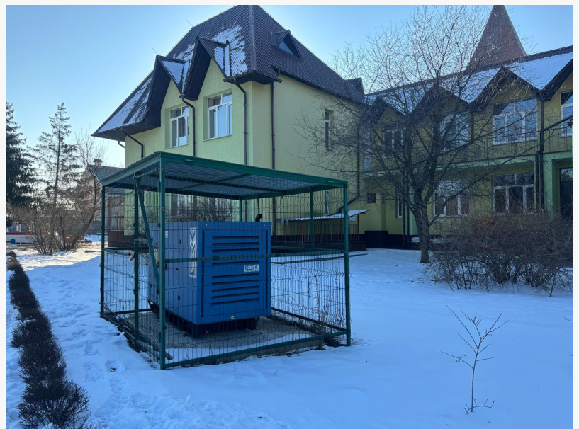
Diesel generator Vorex donated to Ukraine kindergarten
