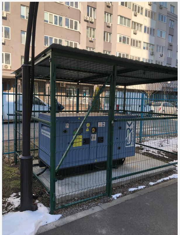
Diesel generator Vorex donated in Kyiv region
