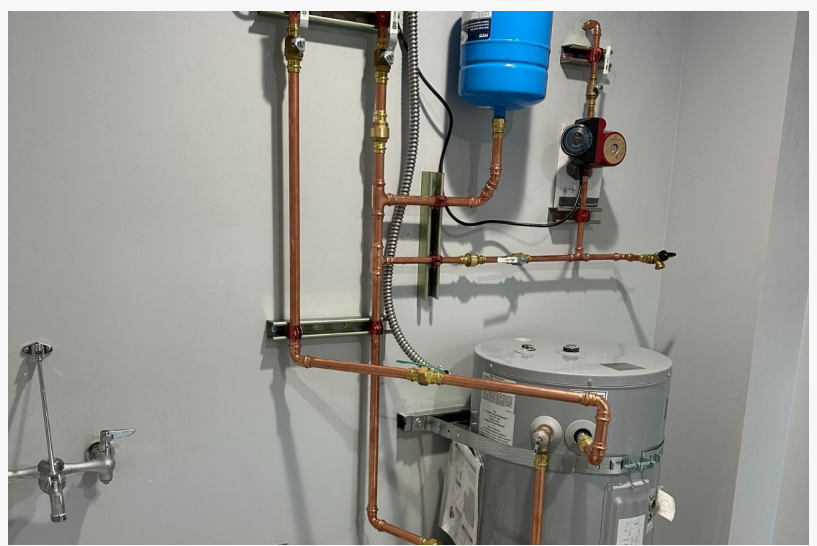
A high-performance water heater system designed for optimal energy efficiency. The installation includes expertly crafted copper piping, an expansion tank, and a circulation pump, ensuring steady hot water flow and pressure control.
