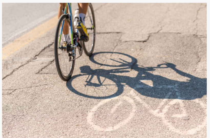
Road bicyclist rides on damaged and deteriorated roadway.
