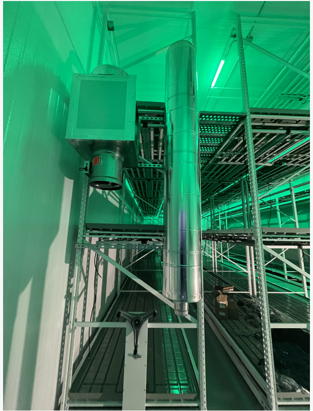
Growing Room: Integrated Racks with Green Lights
