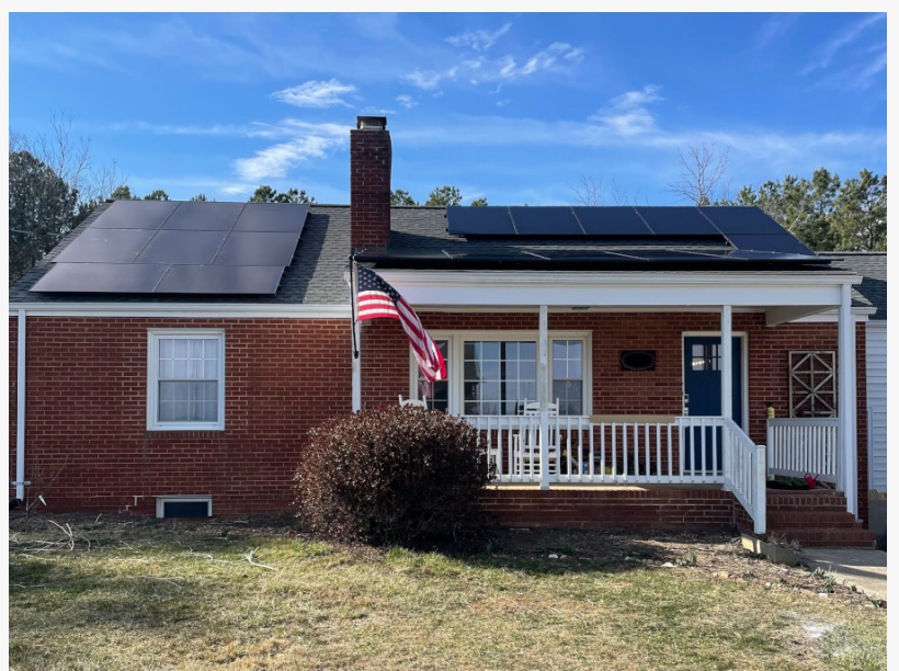
Virtue Solar installs high-quality solar systems & battery backup solutions in Virginia.
