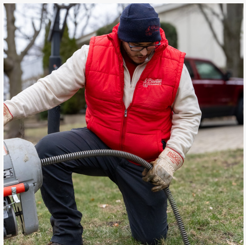
A J. Blanton Plumbing technician conducting a plumbing inspection, helping homeowners prevent hidden dangers of spring thaw with expert plumbing contractors and emergency plumber services.
