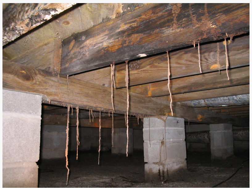
Termite Damage Chesapeake
