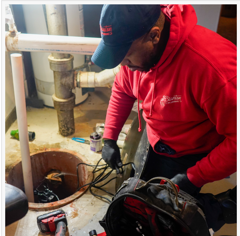
A J. Blanton Plumbing technician repairing a sump pump, ensuring homeowners are protected from basement flooding with expert 24-hour plumbing services this spring.
