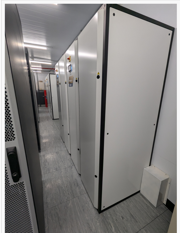
Image from new installation at University of Chichester data centre
