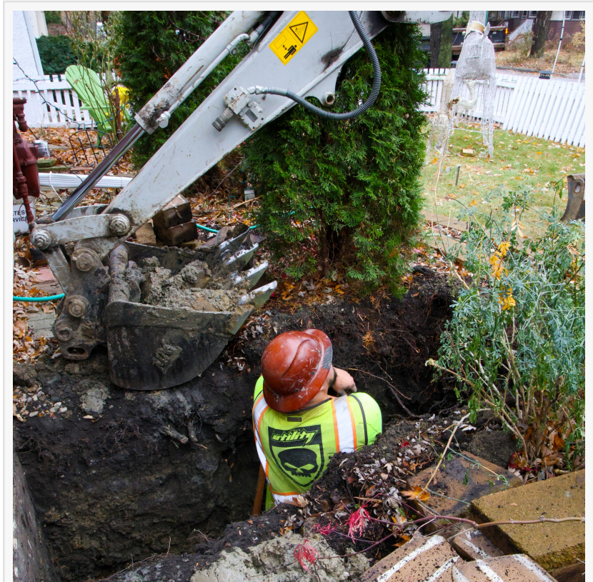
A J. Blanton Plumbing technician performing a plumbing repair, helping homeowners fix pipe damage caused by the spring thaw with expert after-hours plumbing and routine plumbing maintenance.
