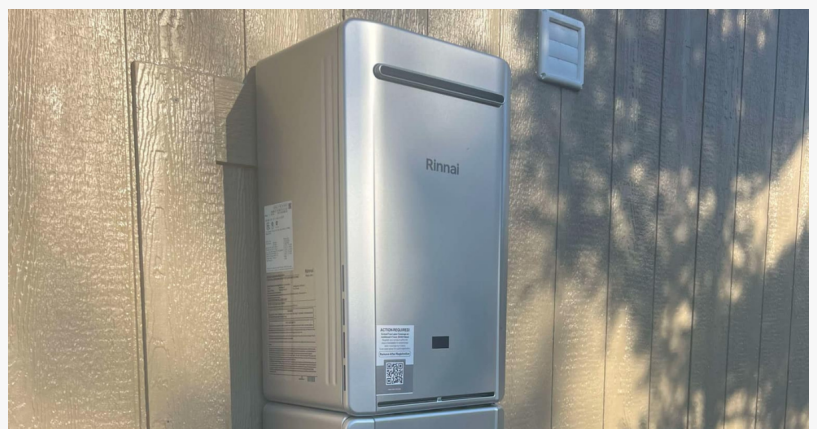
Rinnai tankless water heater installed by the team at Mad Pipers Plumbing.
