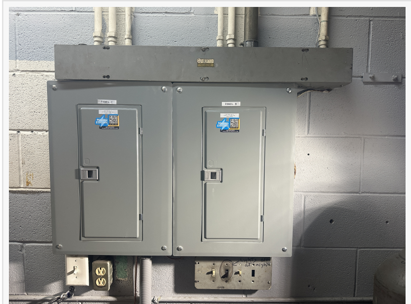
Updated electrical panel installed by Mauro Electric Inc.
