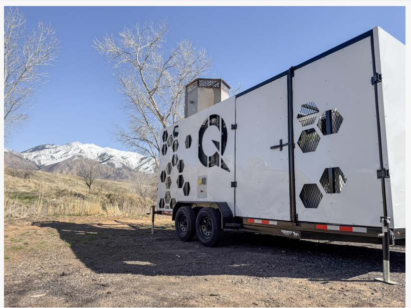
TORCH4 installed and operating at a closed landfill in Weber County, UT
