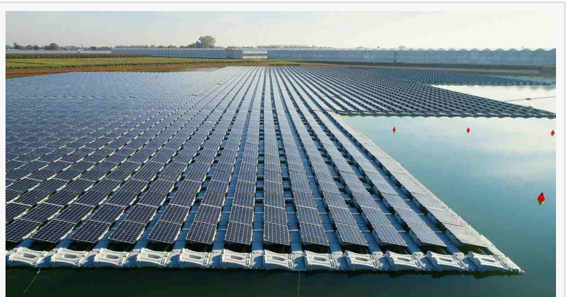
Floating Solar Panels
