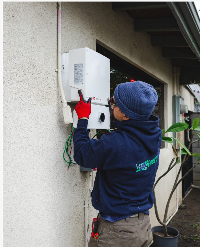
Solar and battery monitoring and maintenance
