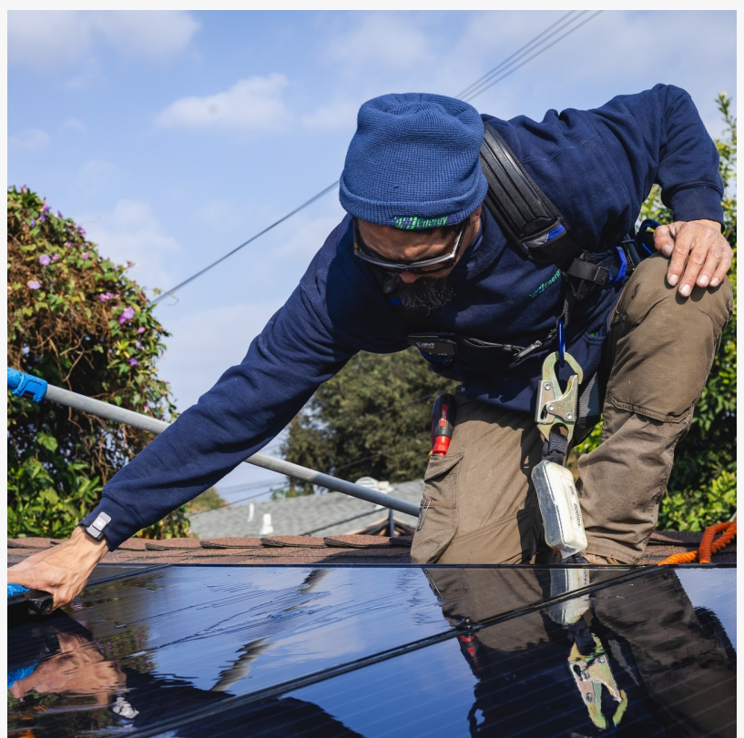
Solar panel cleaning
