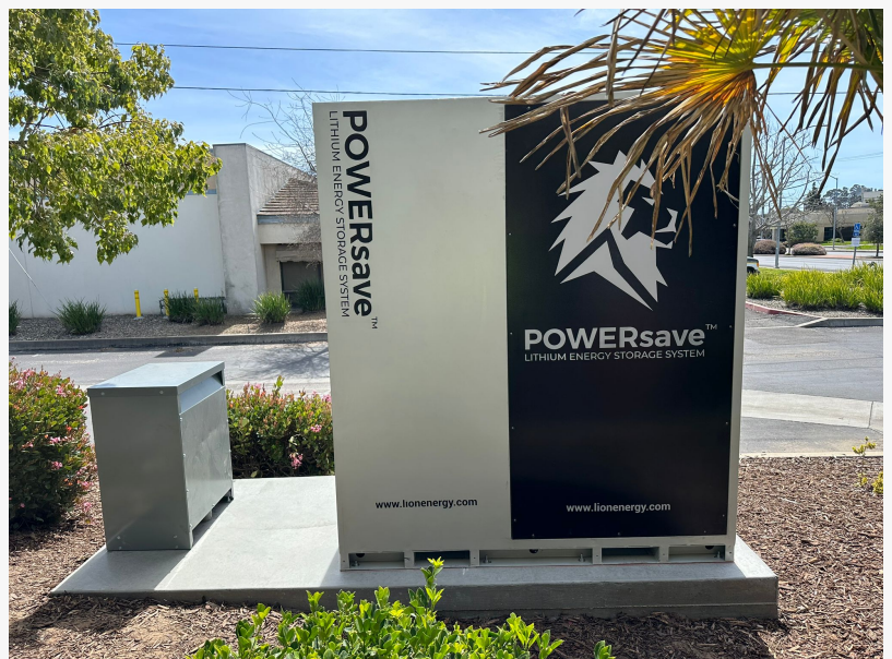
Simmitri Commercial Battery Installation
