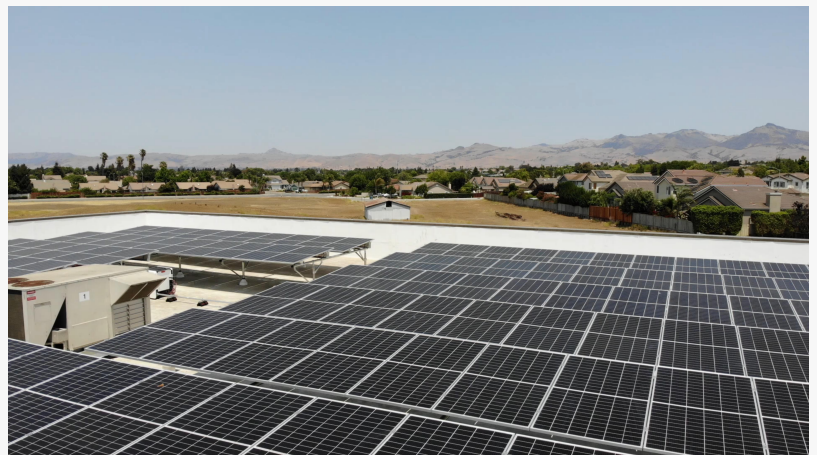
Simmitri Inc. Commercial Solar Installation
