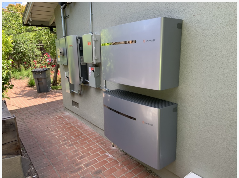
Simmitri Inc. Solar Battery Installation
