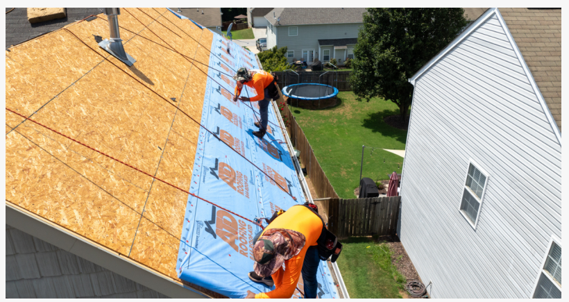
The ATD Roofing crew works efficiently and securely to protect what matters most—your home.
